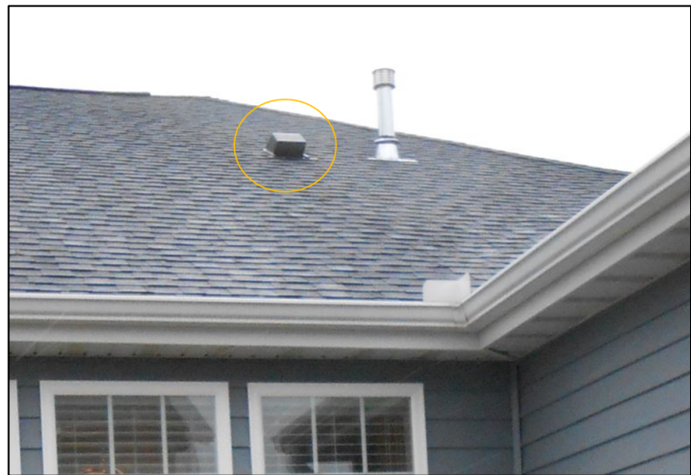
P2. Exhaust fan vent (circled). A cap like this shows that the fan attached is exhausting to outdoors.
