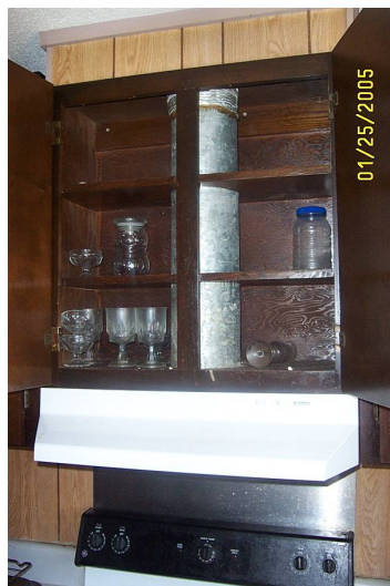
P1. Duct for a range hood. Without a duct, air does not leave the house.
