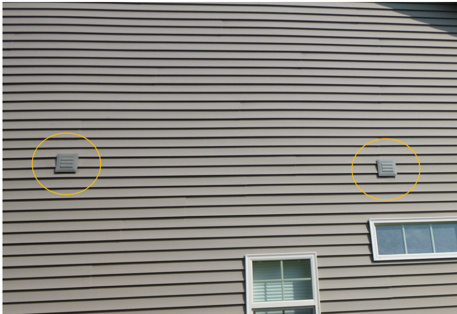
P3. Exhaust fan vents through the wall (circled). Each one could be connected to a fan with a duct, showing that the fan is venting outdoors. One of the vents might be for a dryer.
